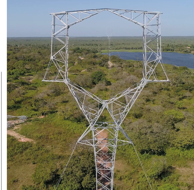
Electricity tower of the Brazilian company Argo, which is in the process of being acquired
