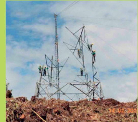
Construction work of tower 309, second section of the Tesalia - Alférez project in Pradera, Valle del Cauca
